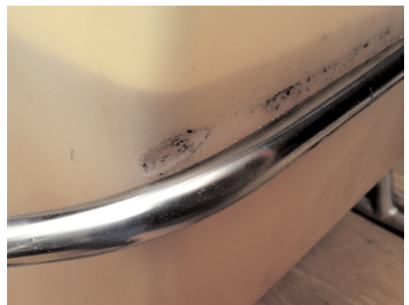
Fig 2 The same tank showing significant wear.
